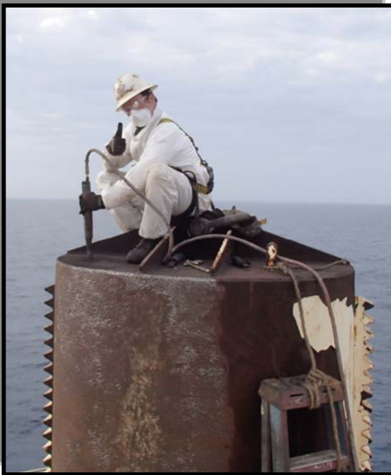
Austin Rutledge chipping on the stern leg tip on the M/V RAM XII.
