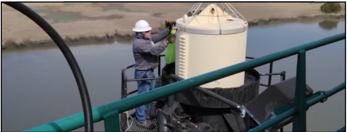
Paul Bourque installing bird safety device on the top of the RAM VII
